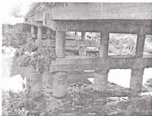
Figure 1.4: Combined Effect of Local and Contraction scour to the Pier and abutment: Balaju bridge and Gongabu bridge respectively.
